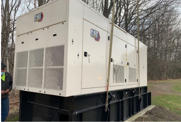
(New CAT 500 kW generator purchased by the Town. The generator was installed on the Barre Town Middle and Elementary School property during the summer of 2021)
