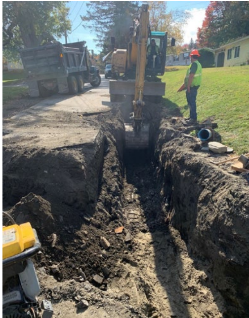
Public works employees Zack LaPerle (operating the town's backhoe) and Brandon Guyette (overseeing digging) are working on installing the new waterpipe line on Littlejohn Road.
